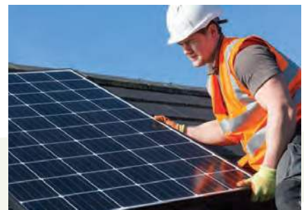
Solarcentury installs solar systems for IKEA customers in Germany
