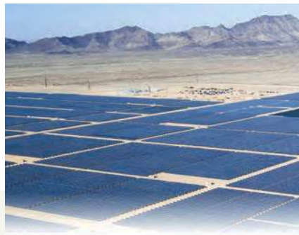
Kinematics solar tracking systems rotate ground-mounted solar panels
