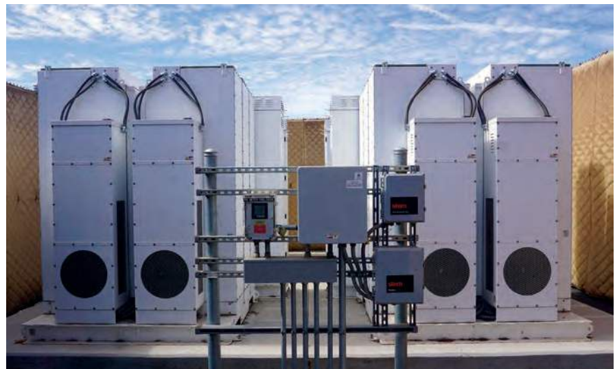
Stem 1.25 MWh battery system installed at a school in Southern California.
