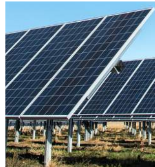
North Sun Solar
