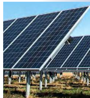
North Sun Solar
