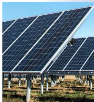
North Sun Solar
